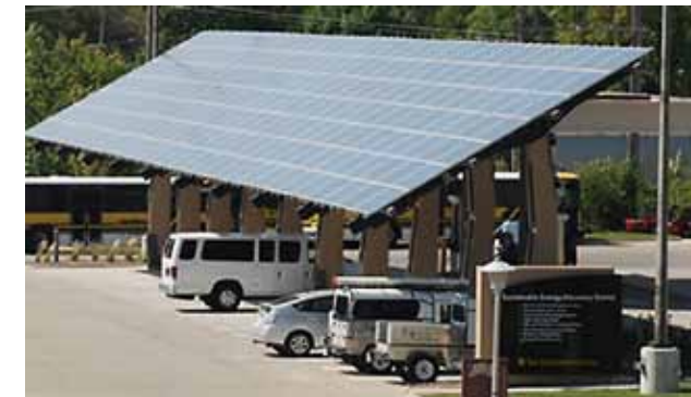
This solar e-car charging station on the campus of the University of Iowa provides charging spaces for approximately 20 electric vehicles for Facilities Management and other departments. The project was completed in summer 2011.
