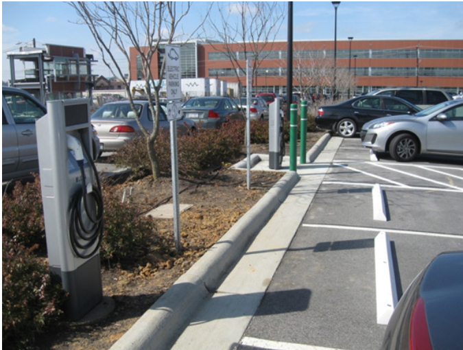
Figure 2. Charging stations at the Durham County Human Services Complex, Durham, NC
